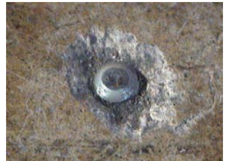
Damaged floor with remains of traditional anchor
