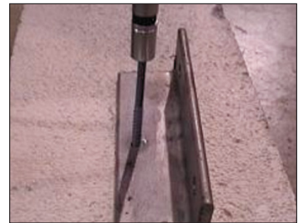
3. Place head of anchor in hex socket, positioning the anchor in the drilled hole, and drive anchor until anchor is fully seated.
